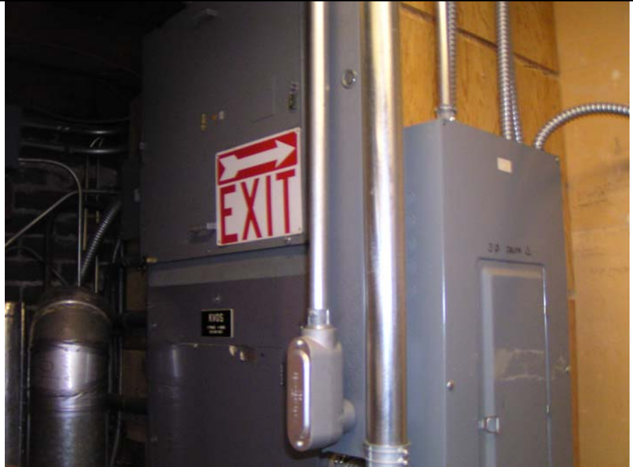
Main Electrical Service
