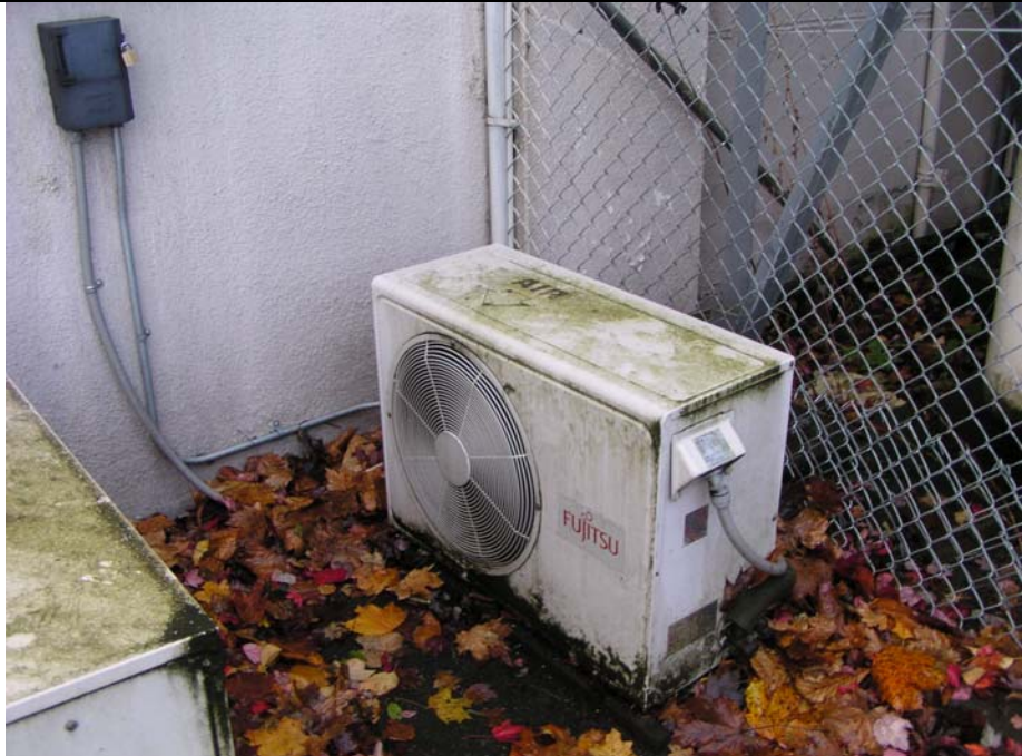
Ground unit next to antenna tower
