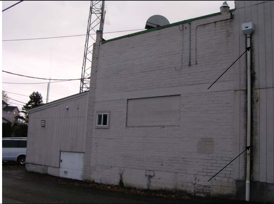
Exterior wall rotting
