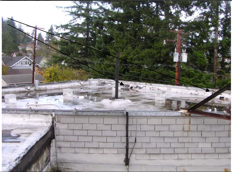
Roof – Problematic scuppers at right
